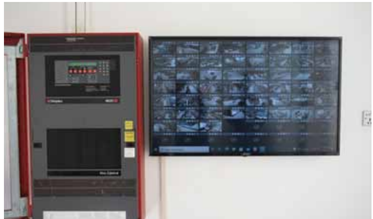
Fire Control and CCTV Monitoring Room
