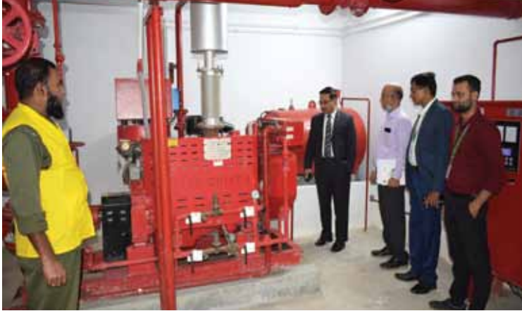
Fire Pump Room
